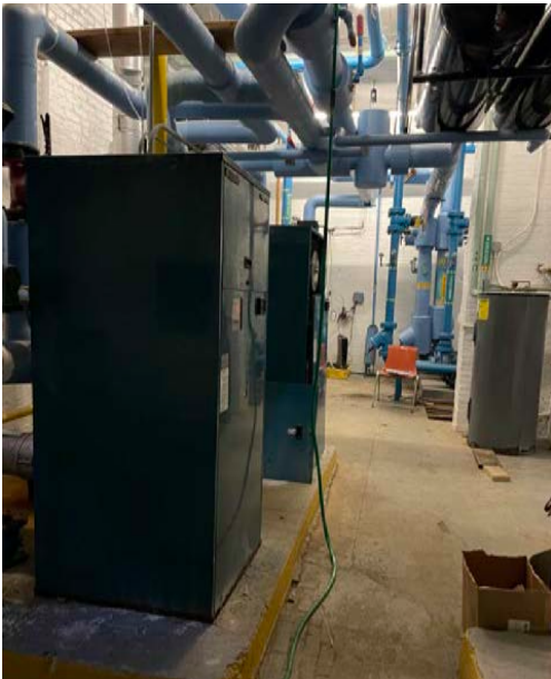
Existing mechanical room
